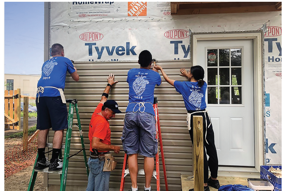
HOUSING SUPPORT: Members of the Human Dimension course help a local builder install vinyl siding on the home of one of the families participating in the program.
